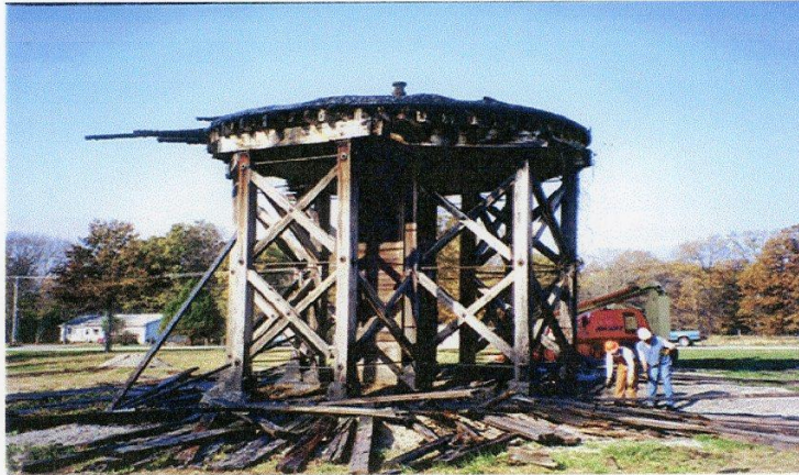
STAVES AROUND BASE OF TOWER
